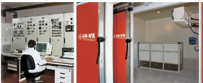
Dooble cold rooms laboratory
